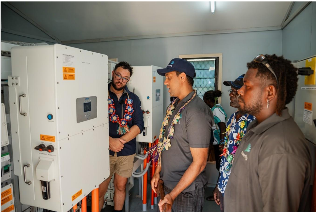
Caption 1: Gavin Peirera from Superfly showing AHC First Secretary Infrastructure - John Hutton and Constituency Project Officer, Dever Daga how the Solar Hybrid Power Systems works.
